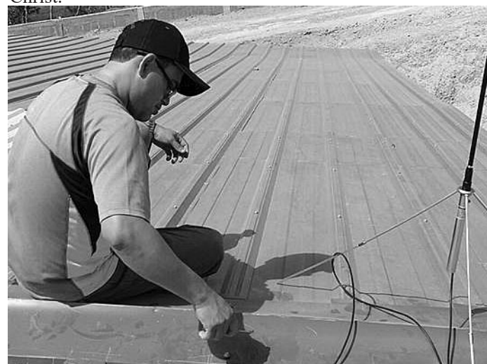
A LifeWord Community Radio transmitter is installed in Diriomo, Nicaragua by a media trainee
